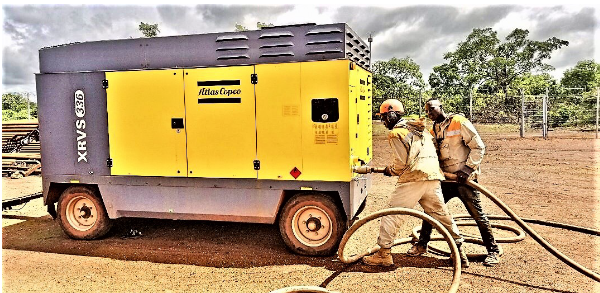
Figure 4.3 Special equipment (high pressure compressor Atlas Copco)
